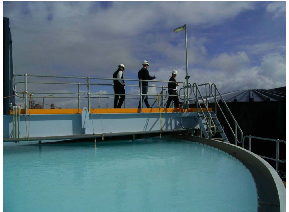
Lime clarifier, Perth.
